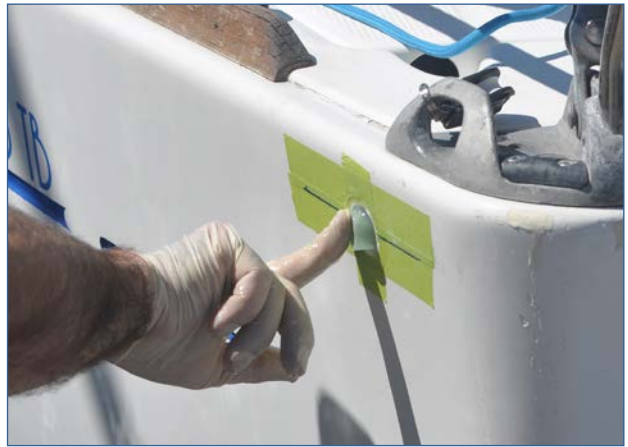
Fig 10: Make sure that there is a proper bond without voids or gaps.
